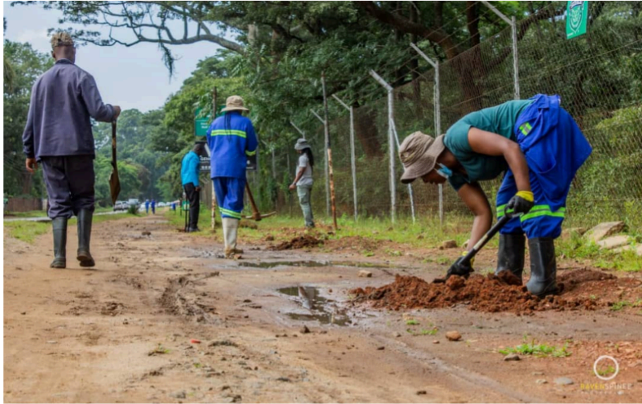
Harare City Council workers constructing a cycle lane along Ridgeway road in Harare Zimbabwe. Image used with permission by Jenna Hutchings.
